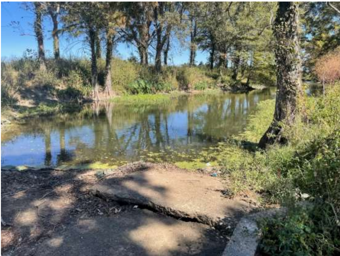
Photo B4: Downstream view across the Tensas Bayou Weir (taken by Thomas Van Biersel on 10/19/22).
