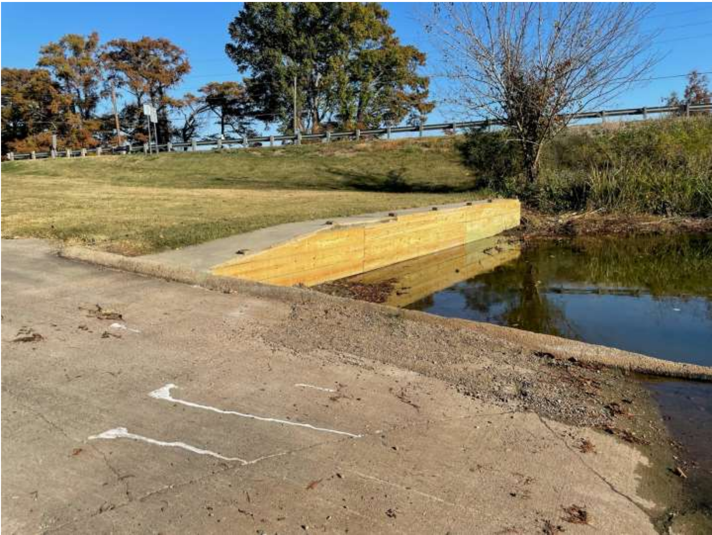
Photo A4: Finished repair at the Tensas Landing boat launch. Photo taken 10/17/2022 by Francis Lensing
