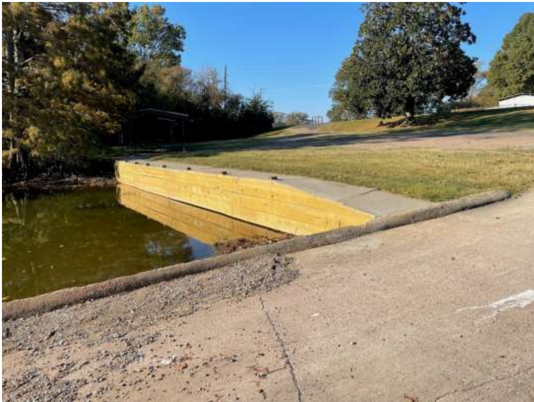
Photo A2: Finished repair at the Tensas Landing boat launch. Photo taken 10/17/2022 by Francis Lensing.
