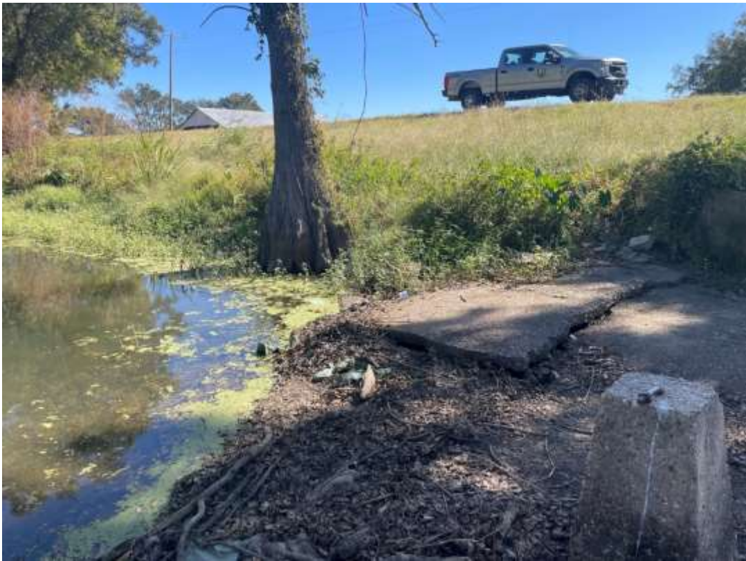
Photo B8: Downstream view across the Tensas Bayou Weir. Notice the dislodged front apron (taken by Thomas Van Biersel on 10/19/22).
