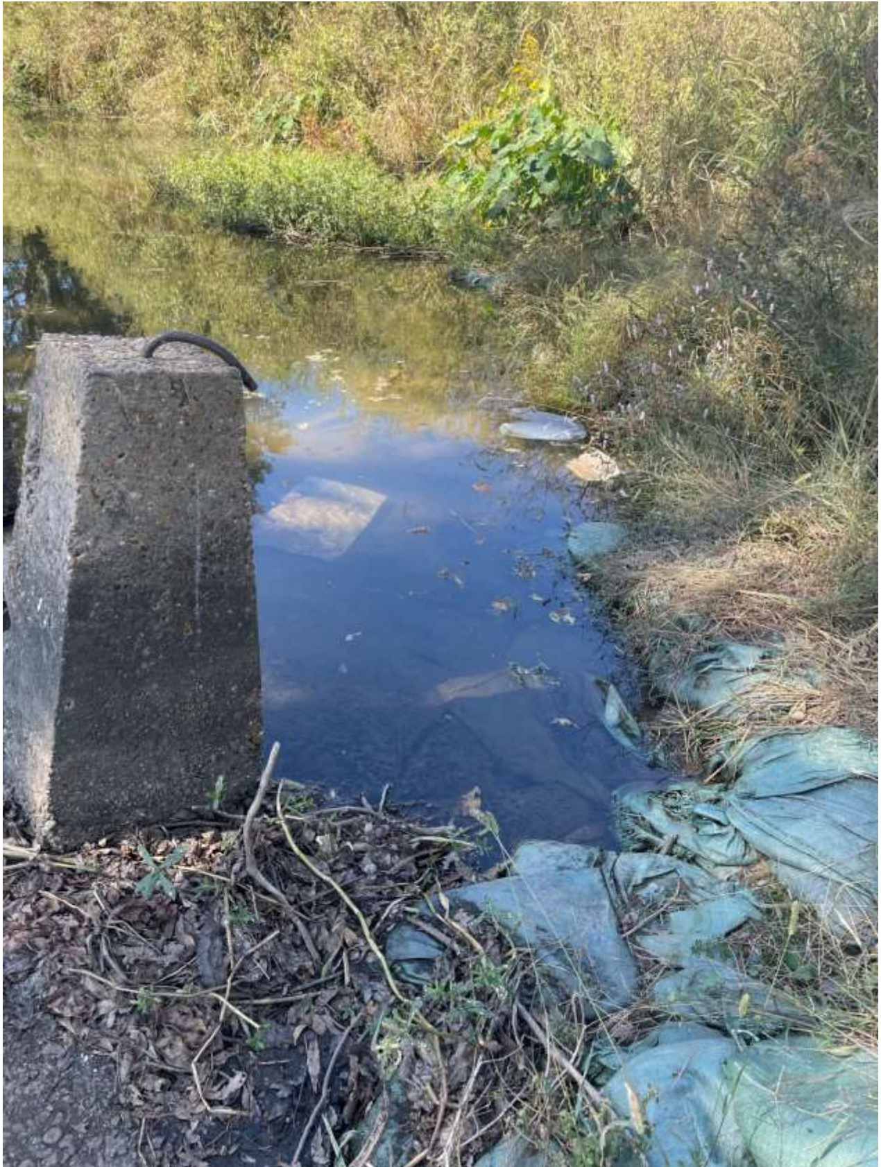
Photo B9: Downstream view across the Tensas Bayou Weir. North edge of the weir where water bypass the structure (taken by Thomas Van Biersel on 10/19/22).
