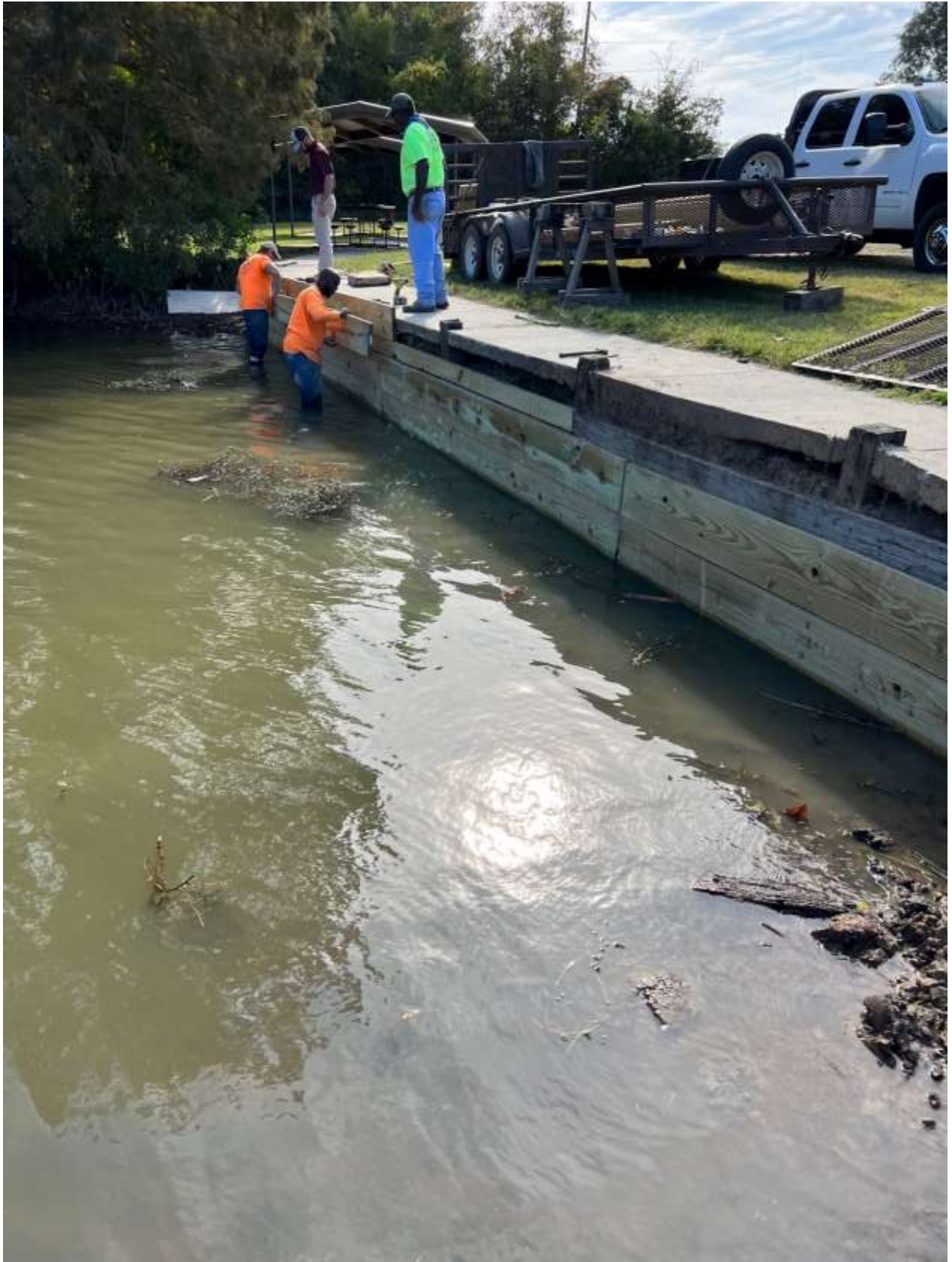
Photo A3: On-going repair at the Tensas Landing boat launch. Photo taken 10/17/2022 by Francis Lensing
