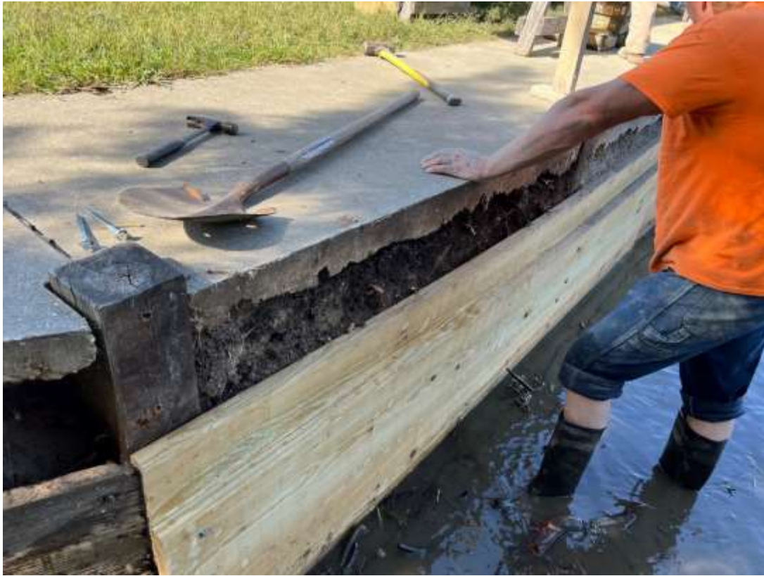
Photo A1: On-going repair at the Tensas Landing boat launch. Photo taken 10/17/2022 by Francis Lensing
