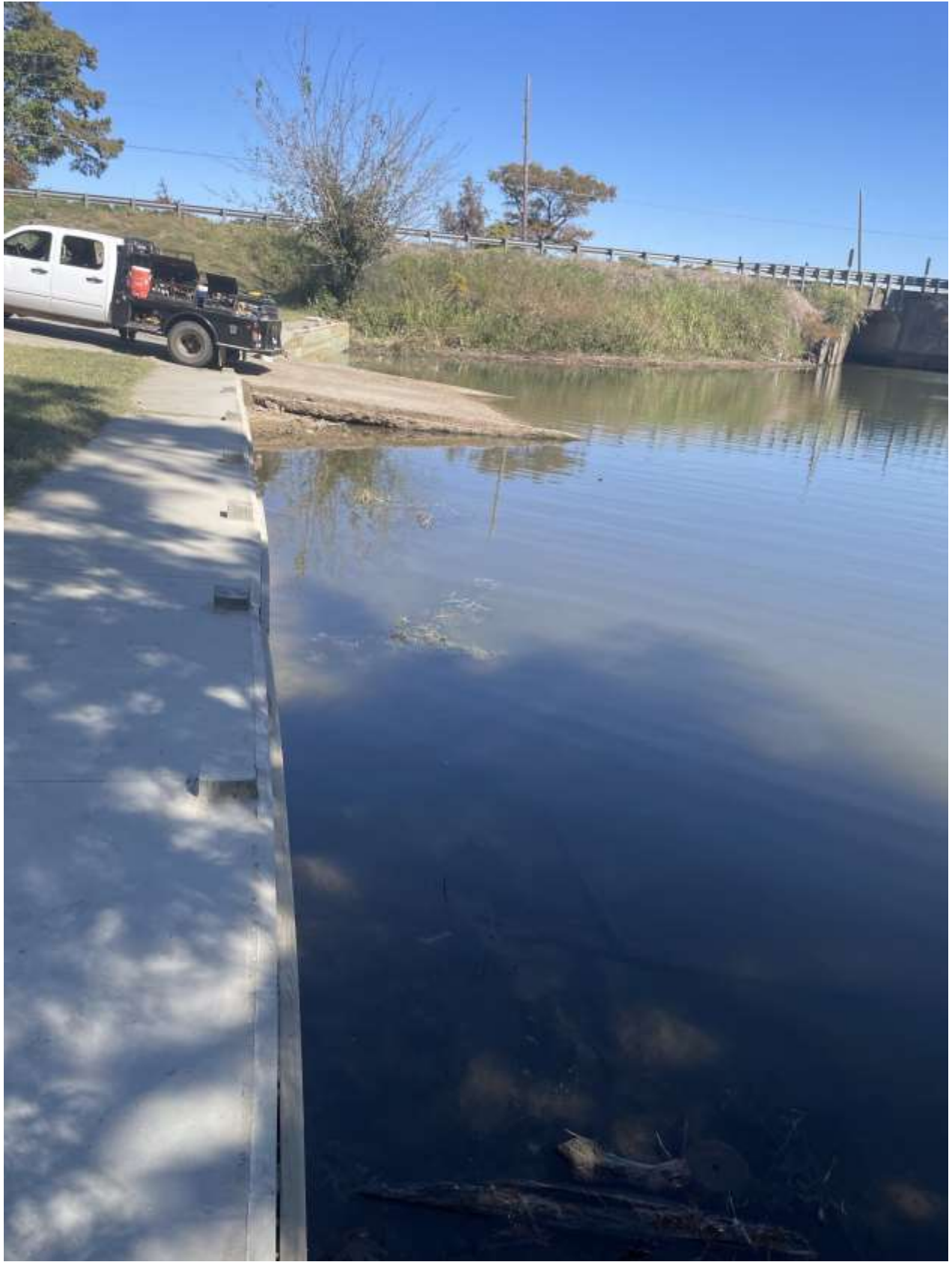
Photo A5: Finished repair at the Tensas Landing boat launch. Photo taken 10/19/2022 by Thomas Van Biersel
