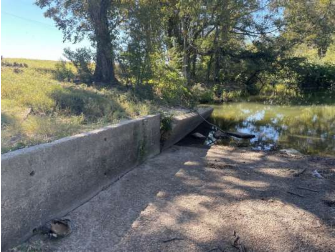
Photo B7: Downstream view across the Tensas Bayou Weir (taken by Thomas Van Biersel on 10/19/22).
