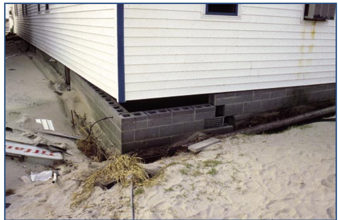
Failure of crawlspace foundation undermined by scour.
