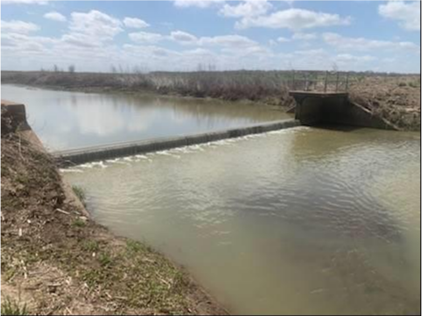
Photograph E3: View southeast across the Baxter Bayou Control Structure (taken by Roger Clement on 3/29/22).
