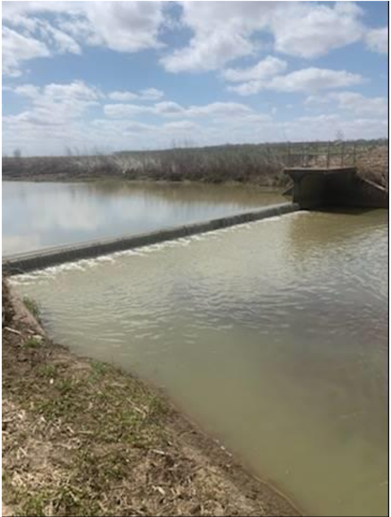
Photograph E1: View southeast across the Baxter Bayou Control Structure (taken by Roger Clement on 3/29/22).
