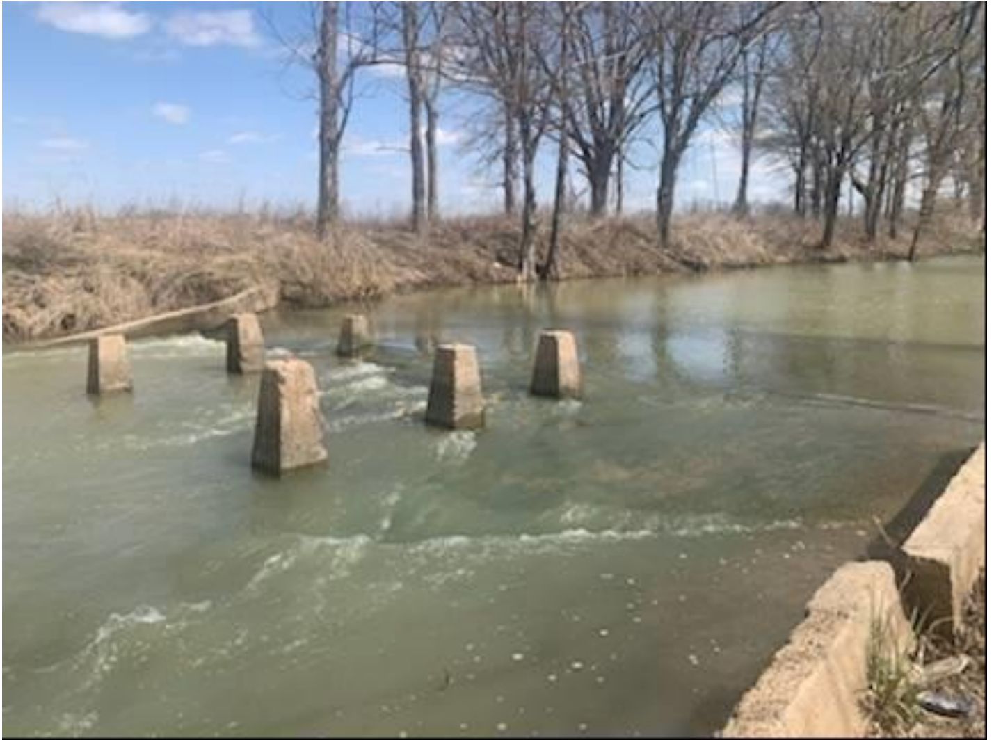
Photograph C3: View north across the Tensas Bayou Weir (taken by Roger Clement on 3/29/22).
