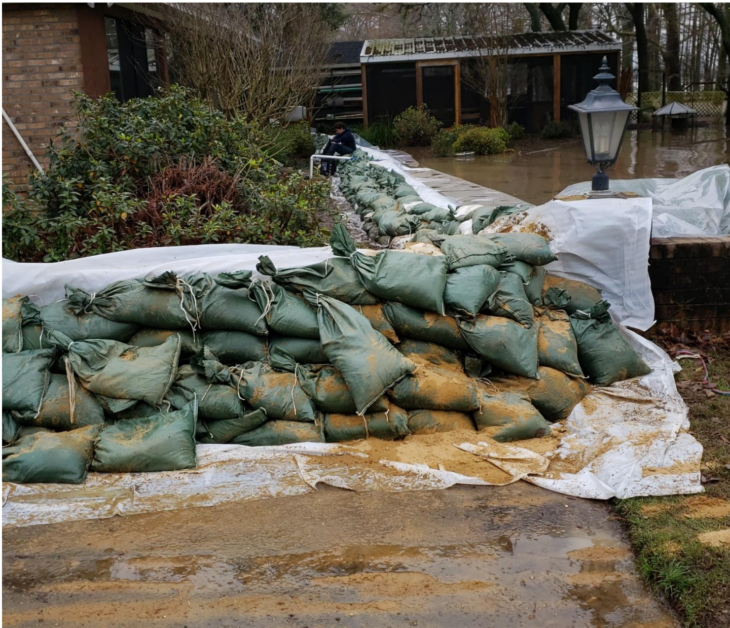
Photo A4: Sandbagging at the residence of 506 Island Point Dr which is the north end of Lake Providence. Photo taken 6/12/2021 by Reynold Minsky.
