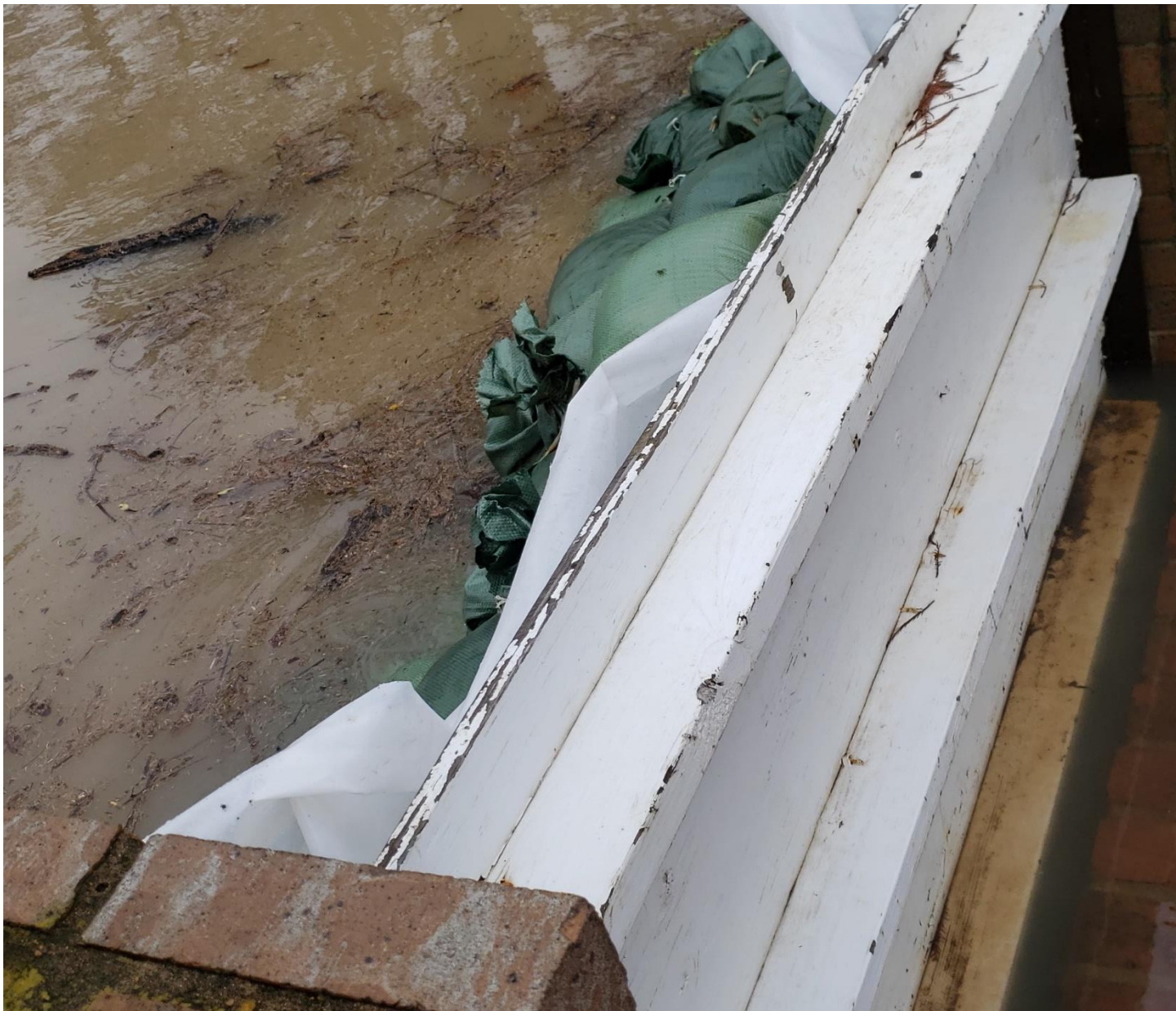
Photo A8: Sandbagging at the residence of 506 Island Point Dr which is the north end of Lake Providence. Photo taken 6/12/2021 by Reynold Minsky.
