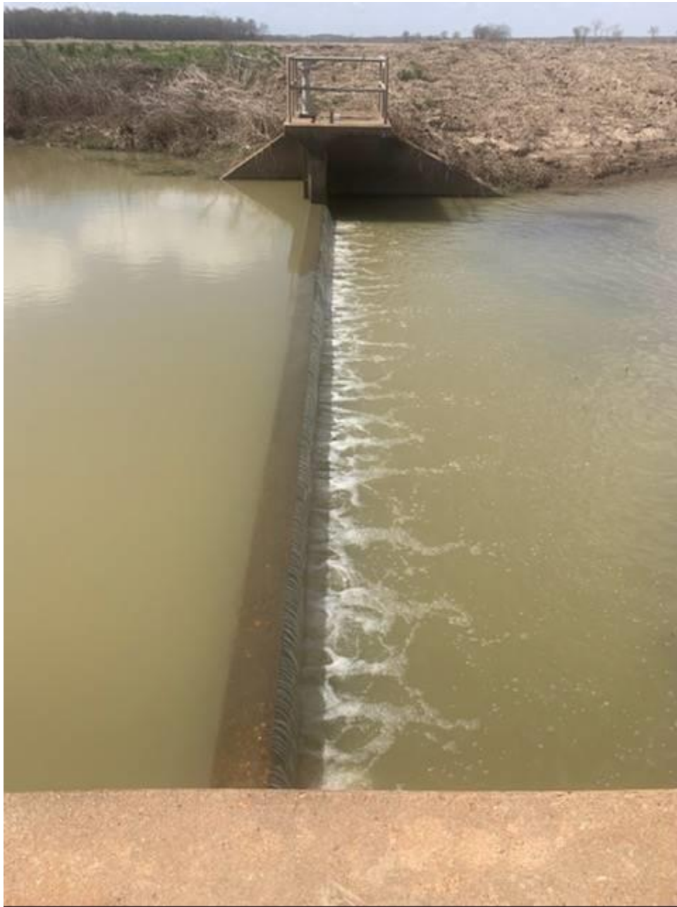
Photograph E2: View south across the Baxter Bayou Control Structure (taken by Roger Clement on 3/29/22).
