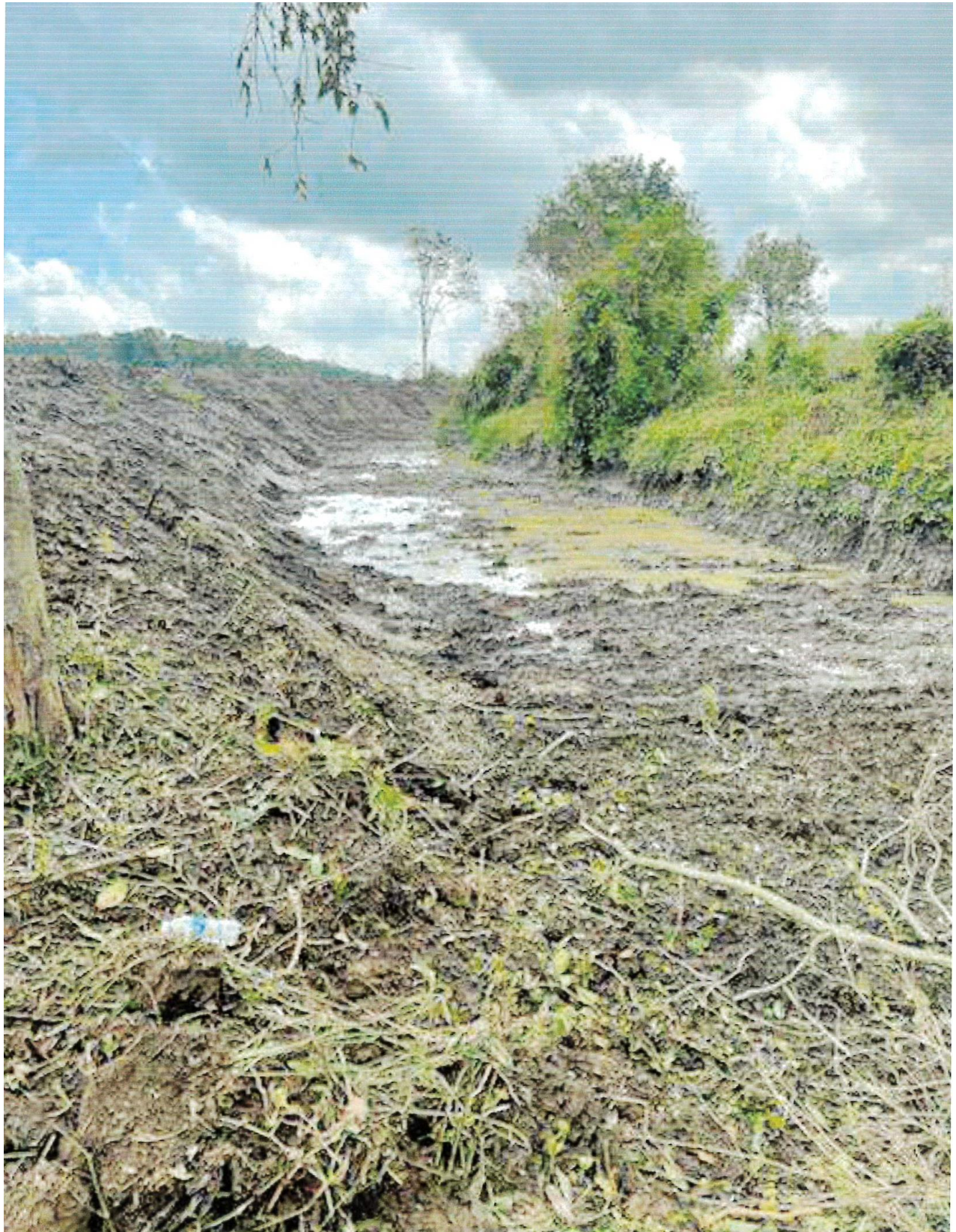
Photo B6: Area near Baxter Bayou structure on September 18 th . Photo taken on 9/18/21 by Bo Holt.
