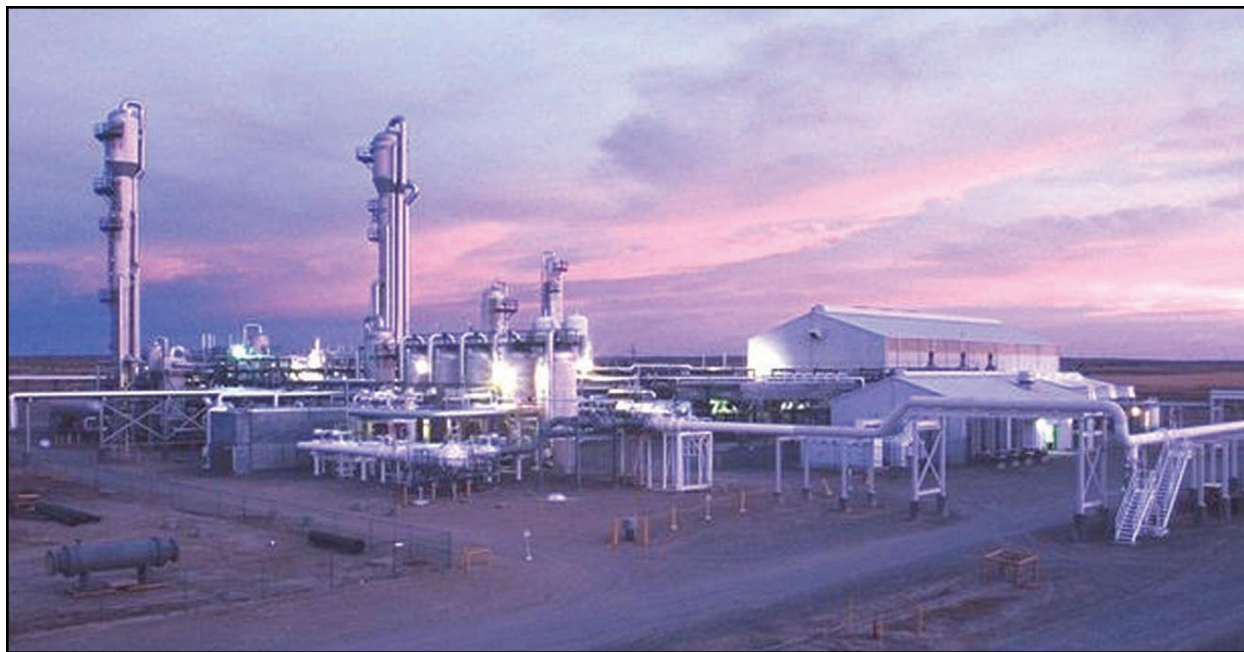
Enterprise Natural Gas Processing Plant
